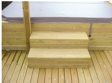
Steps up to a hot tub constructed from decking boards and stringer underneath
